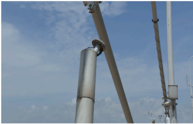
Fig. 8. Damper bolt fell off from cables.
